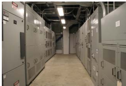
The three variable frequency drives allow us to test 50 and 60 HZ units.
