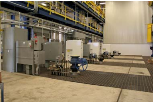
Pictured are the control cabinets located at each test stand.
